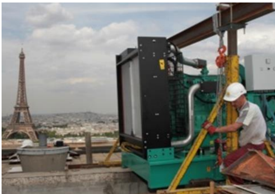
Figure 2. Temporary power source with 6.7 litre diesel engine used in a construction site. Dirt and dust are an issue at these locations.
